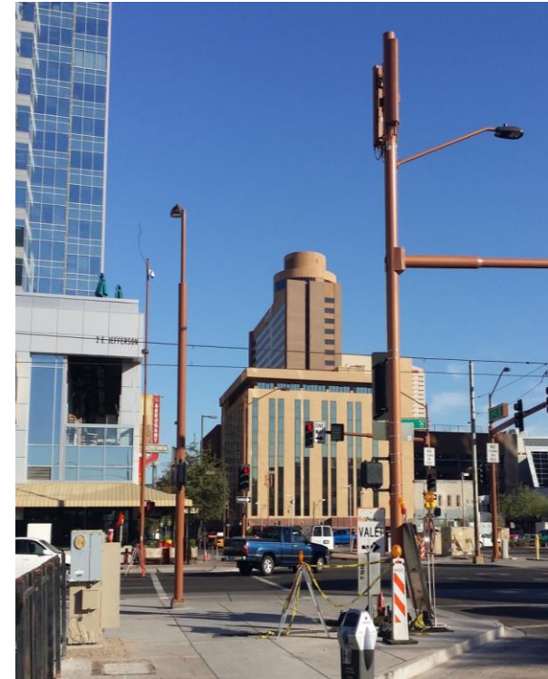
Traffic Control Pole with Cabinet
